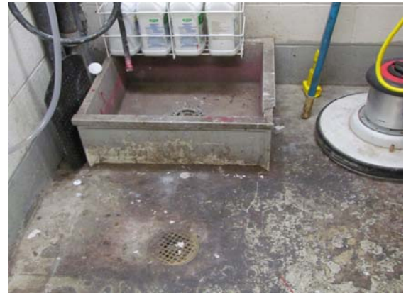
Plumbing issues are a constant maintenance challenge.
