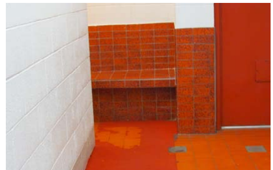
All inmate showers leak and need to be repaired.
